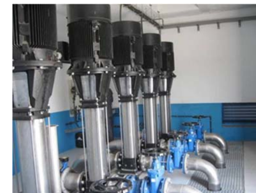
Interior Central ETAP
